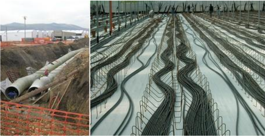
Tubes going from the power plant to the greenhouse.
